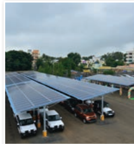
Solar power at a vehicle depot in India, making good use of the car port roofspace
