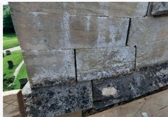
Hollow and insecure stones section found during inspection
