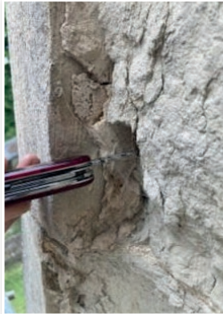
Totternhoe Clunch stone is friable and in poor condition in several areas inspected
